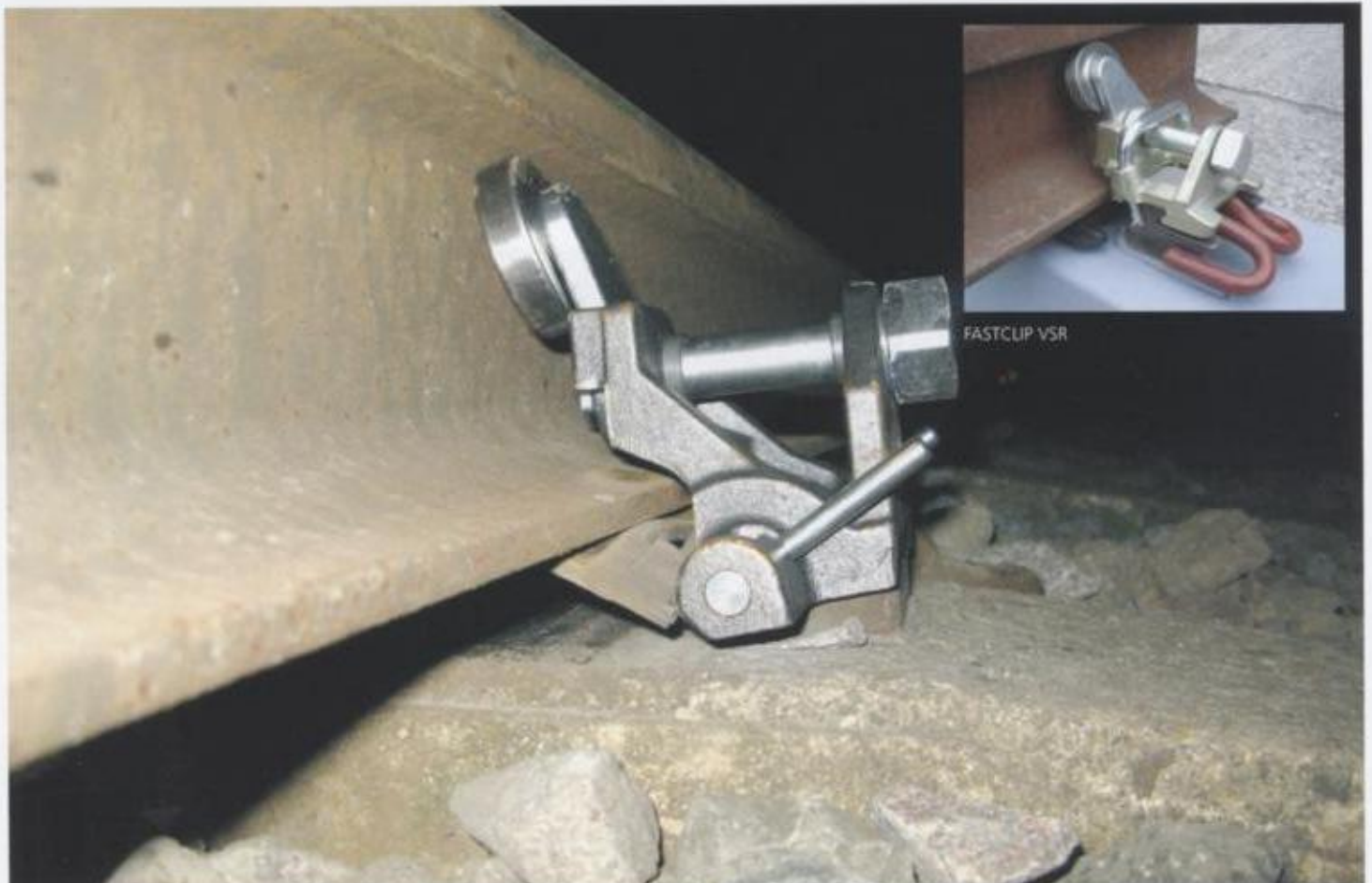
eVSR at Croby Glen in raised position
